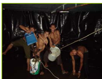
Above: Cleaning the water tank, the liner had a tear and couldn't be repaired. A new liner was sent up in the container. (See container story page 4)
